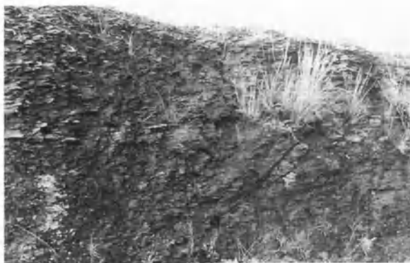
Fig. 8.10. A 3-m section through the Clare Shales showing angled joints, the main mode of transmission of groundwater
