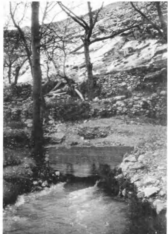
Fig. 3.5. Harouch-Figeh System. Water supply for city of Damascus. Albion Dolomitic limestone (photograph by P. E. LaMoreaux 1980)
